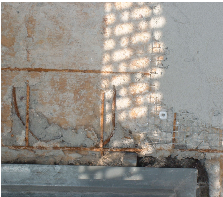
Armanet protection on bad undergrounds
